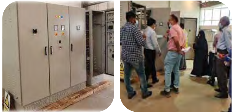
FAT for the Supply of Electrochlorination Rectifier to SEWA - Layyah Power Station
