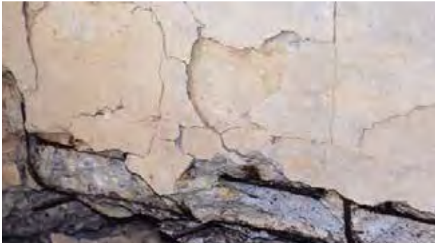
The inevitable end result of all rebar corrosion is concrete damage.
